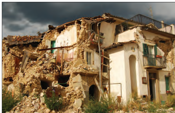
Big impact Building damage in the village of Onna, near L'Aquila in Italy, caused by the April 2009 earthquake.
